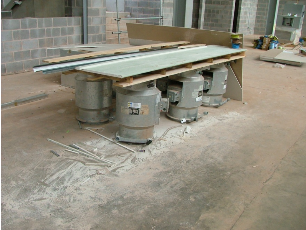
Figure 3: Air-handling units used as a work bench
