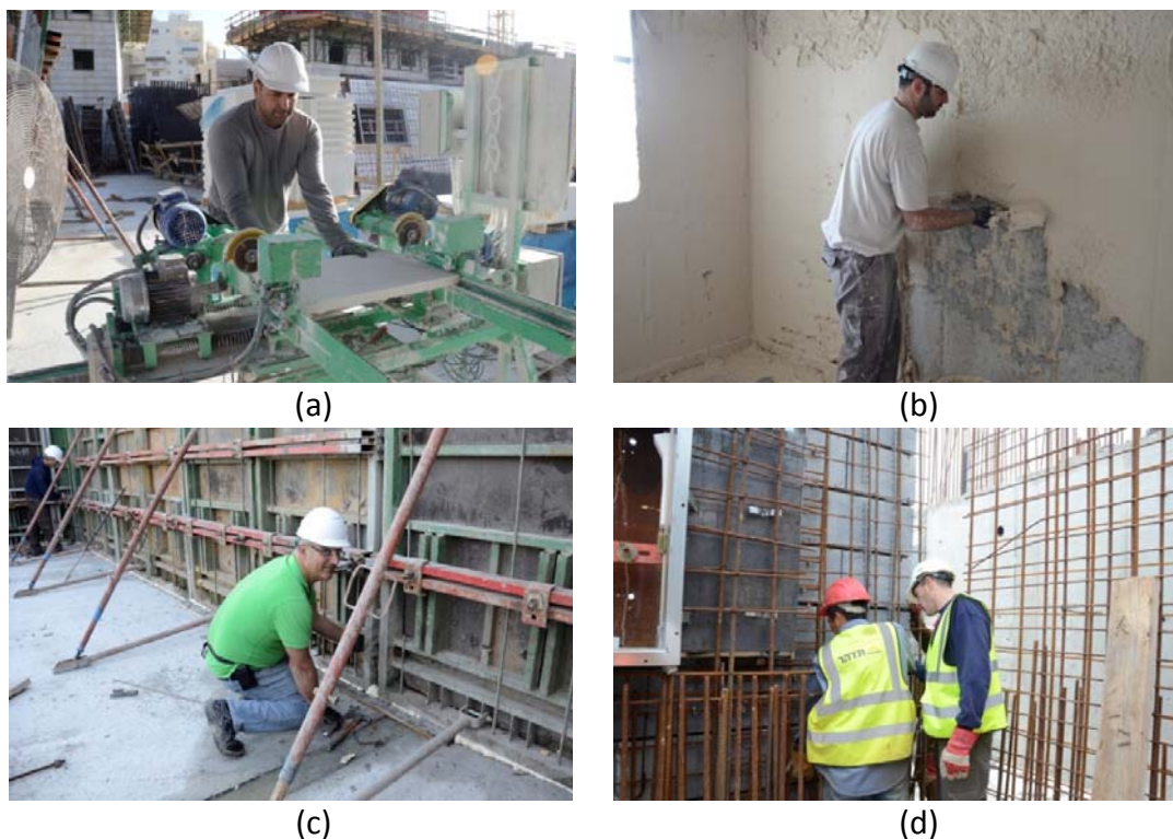
Figure 2 – Managers working in Gemba: a) A project manager preparing stone cladding. b) A project manager applying plaster. c) A logistics manager fixing formwork. d) Tidhar's CEO fixing rebar.
