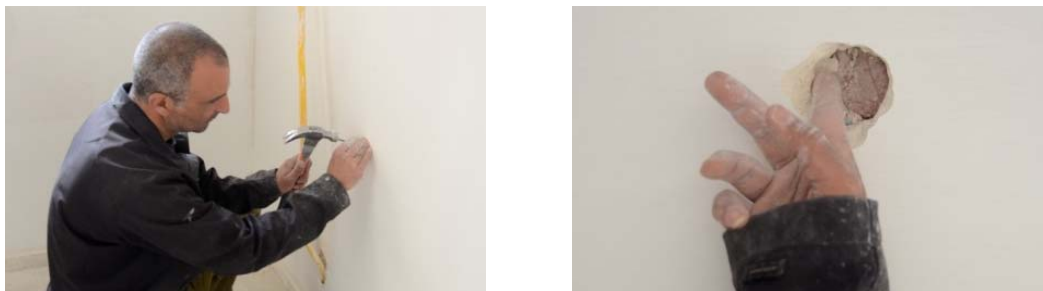
Figure 6 – Revealing electrical outlet boxes: finding the box with a nail (left); removing the plaster around the entire box (right)
